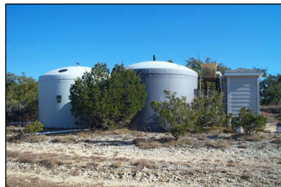
Figure 2-5. Two 10,000-gallon fiberglass tanks
