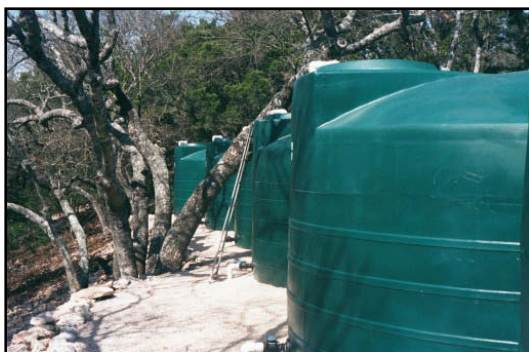
Figure 2-6. Low-profile 5,000-gallon polypropylene tanks
